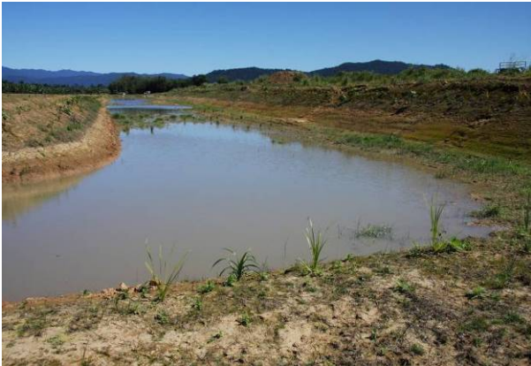
The 2.45 hectare wetland designed and built to treat run-off from the banana farm. Photo: DAFF
